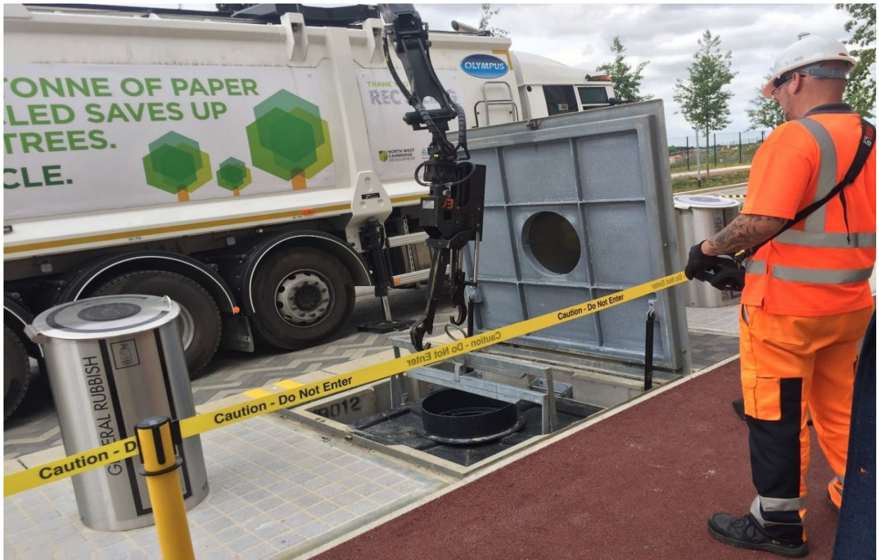
Fig 19 Underground bins hook-lift system in the ground
