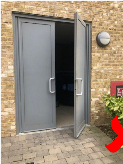
Fig 1 Double doors – do not stay open and will swing shut fast, hindering collections
