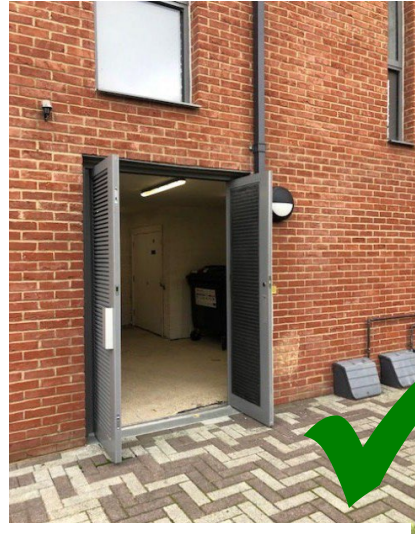
Fig 2 Double doors – stay open while collection takes place, with door bolts, hooks or automatic opening systems
