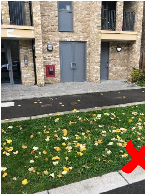
Fig 10 Swales mean there is no smooth access from bin store and bins have to be dragged across grass
